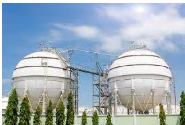
Figure 4: Gas Storage Tanks
